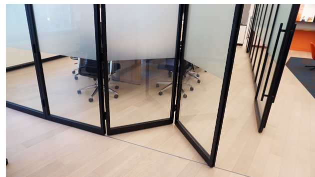
3-WAY INTERSECTION OF PK-30 FIXED GLASS, BI-FOLDING PARTITION, AND SLIDING ENTRANCE DOORS.
